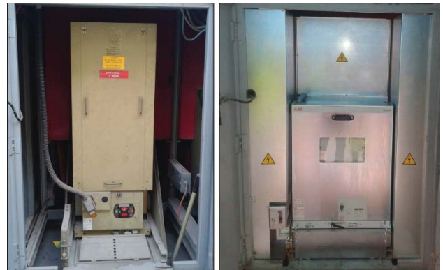
Figure 8. Retrofill of an air magnetic breaker (original at left)
