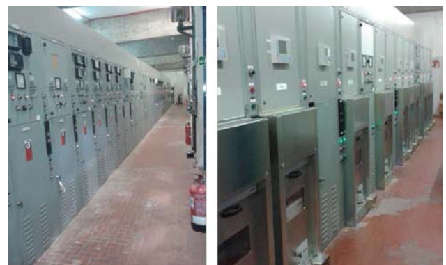
Figure 11. Original switchgear lineup (left) and after retrofill and P&C renewal
