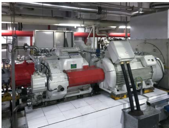
Fig.19 Electro-mechanical ASD installed on a 4.5MW boiler water feed pump
