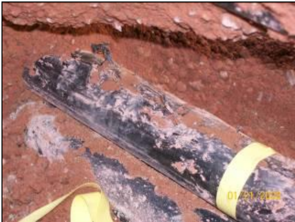
Fig. 4 Cable Damage passing VLF test but pinpointed within 10cm by 50/60Hz PD test
