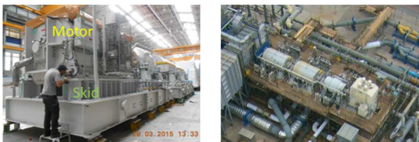
Fig.1. 20MW induction motor integrated on LNG Train [1].
