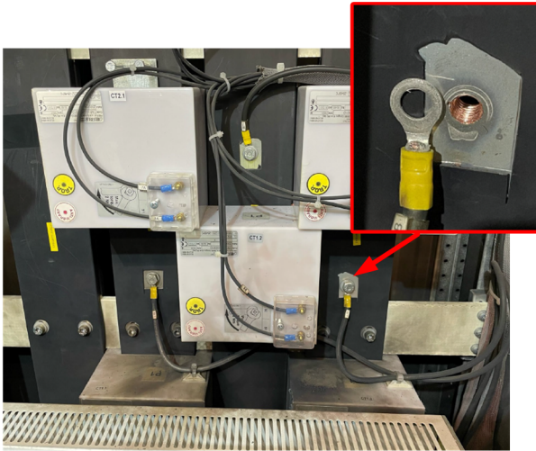
Fig. 21 Postmanufacturing drilled holes on the 380 V busbar
