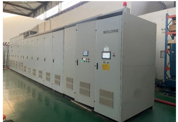
Fig. 3 Cascaded H-bridge inverter ( N=9 ), 10kV, 6MW
