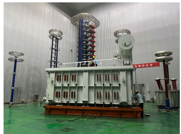
Fig. 13: 55MVA rectifier transformer, secondary outlets for two 6-pulse rectifiers [6]
