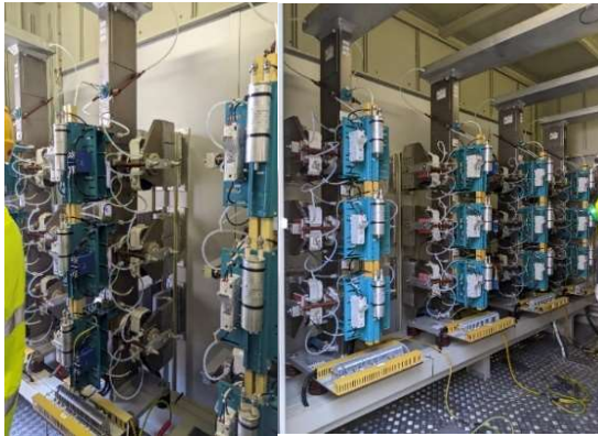
Fig. 24: 2x 16kA rectifier in container housing [6]
