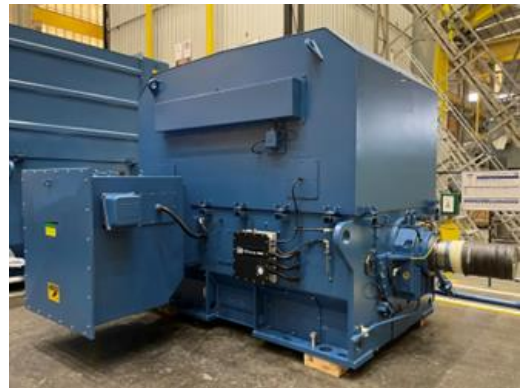
Fig. 2 – Data Acquiring Central Device aspect
