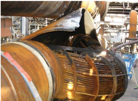
Fig. 4 Effects of Overpressure of Vessel
