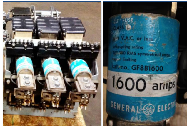
Figure 6: Sample fused power circuit breaker with a current limiting fuse
