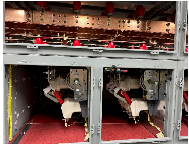
Figure 9 - MV Drive Switchgear - Double Bus and Switch CTM Deployment
