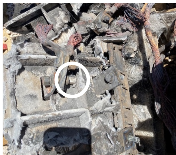
Figure 8 - B-Phase Joint Indicating Loose Connection
