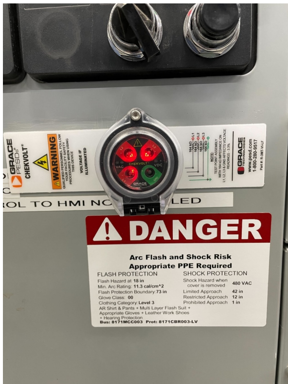
Figure 3 - Panel-Mounted PESD with Illuminated LEDs to indicate Voltage Status
