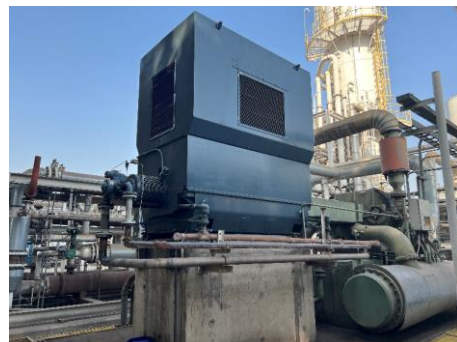
Figure 5. Motor on concrete foundation
