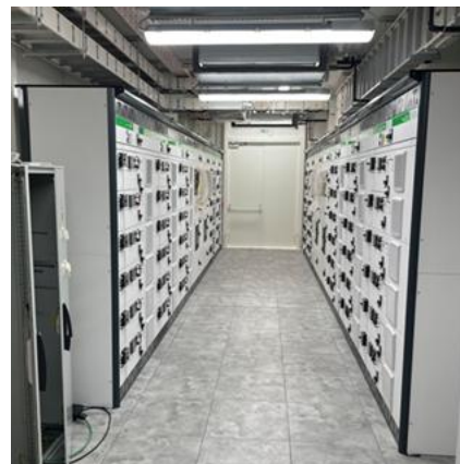
Fig. 25: LV Switchgear with SCR inside substation [9]
