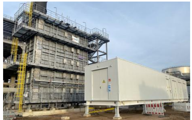
Fig. 24: electrical heater and prefabricated substation [9]
